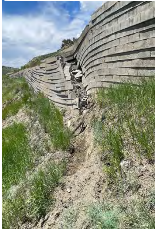
US 50 Cerro Summit Landslide/Wall
